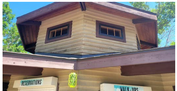
Existing Concessionaires Building Exterior Deterioration
