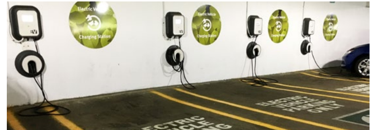
Electric vehicle (EV) charging readiness in single-family homes and methods of EV charging station installation in commercial developments when stations are required by the zoning ordinance
